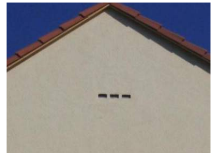
INSTALLED BAT TUBES (X3) WITH A RENDERED FINISH (SOURCE: THE BAT CONSERVATION TRUST WEBSITE)
