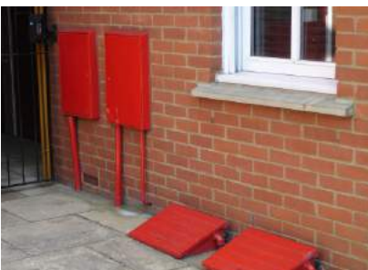
VISIBLE SERVICES BOXES
